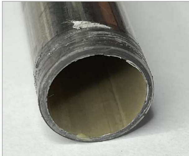
Figure 1. A pipe end covered by grease from the used cutting tool. How can the influence from this on the trend of MIC be evaluated during damage inspection?
